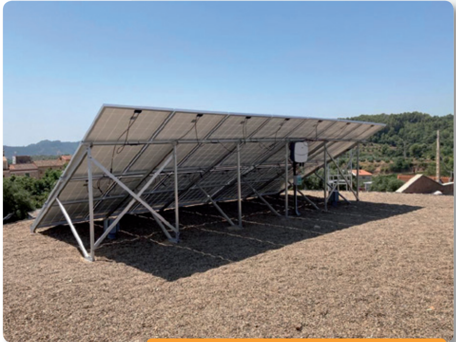
Figura 3. Instalación exterior en Tarragona, España Figure 3. Outdoor installation in Tarragona, Spain
