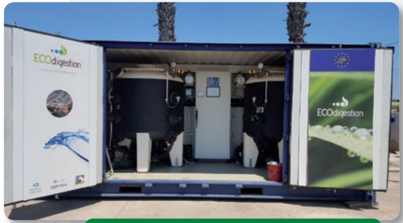
Figura 4. Planta piloto | Figure 4. Pilot plant
